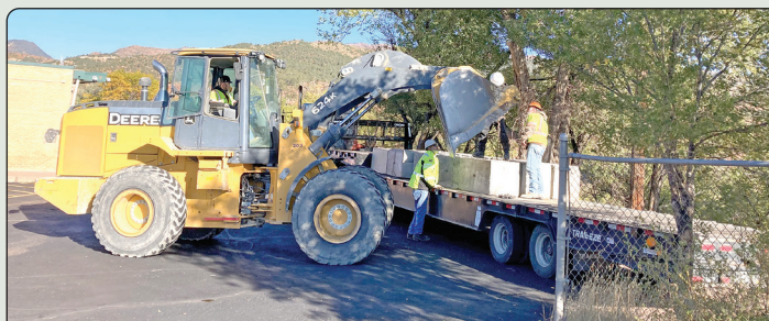
At far left, building materials arrive at the high school. At left, The materials are unloaded using a wheel loader.
